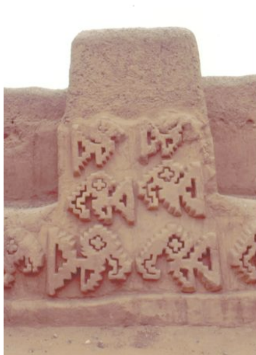
Fig. 03 - Tschudi Palacio, Chan Chan, Peru. Top protection.
