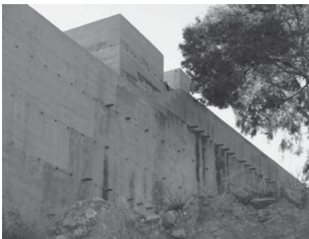
Figure 7. Part of the external wall of the castle of La Mola (Novelda, Alicante, Spain) with the regularization of the volumes (Vegas & Mileto).
